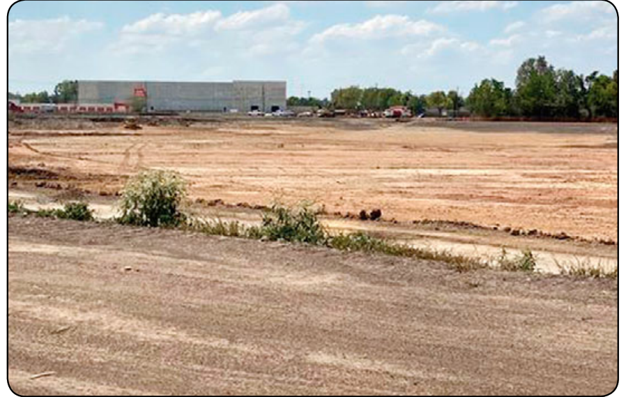
Work continues on the Harris County Flood Control District's South Shaver Stormwater Detention Basin, located near South Shaver and SH 3/Old Galveston Road. Part of the county's 2018 bond program, the new basin will detain around 420 acre-feet, or 138 million gallons, of stormwater. HCFCD and Precinct 2 Commissioner Adrian Garcia's office plan to beautify the basin once complete.
