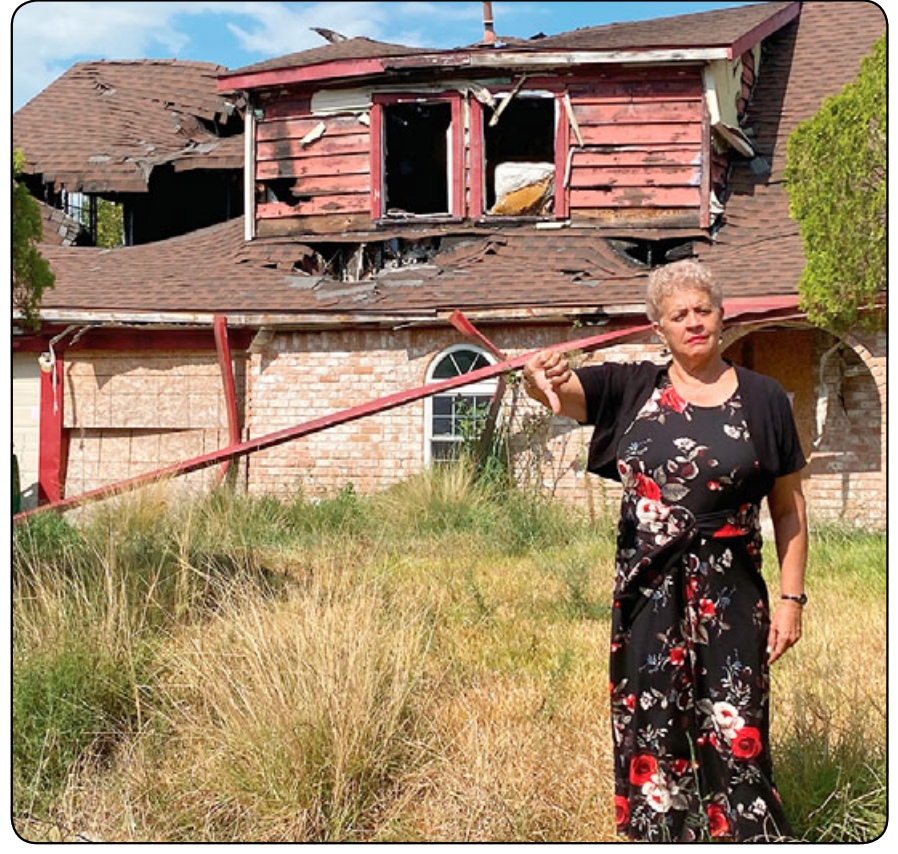
Following two years since a fire destroyed this home on Sageburrow in the Sagemont subdivision, it is set to soon be demolished, thanks to the efforts of the Sagemont Civic Club, District D City Council Member Carolyn Evans-Shabazz (shown giving a "thumbs up") and the Leader. Destroyed by fire in August 2021, the house has been abandoned since the incident and deemed an eyesore and safety hazard by area residents. A second nuisance, a house on Sageheather, abandoned roughly 15 years ago, is also slated to be demolished. Photo by Marie Flickinger
