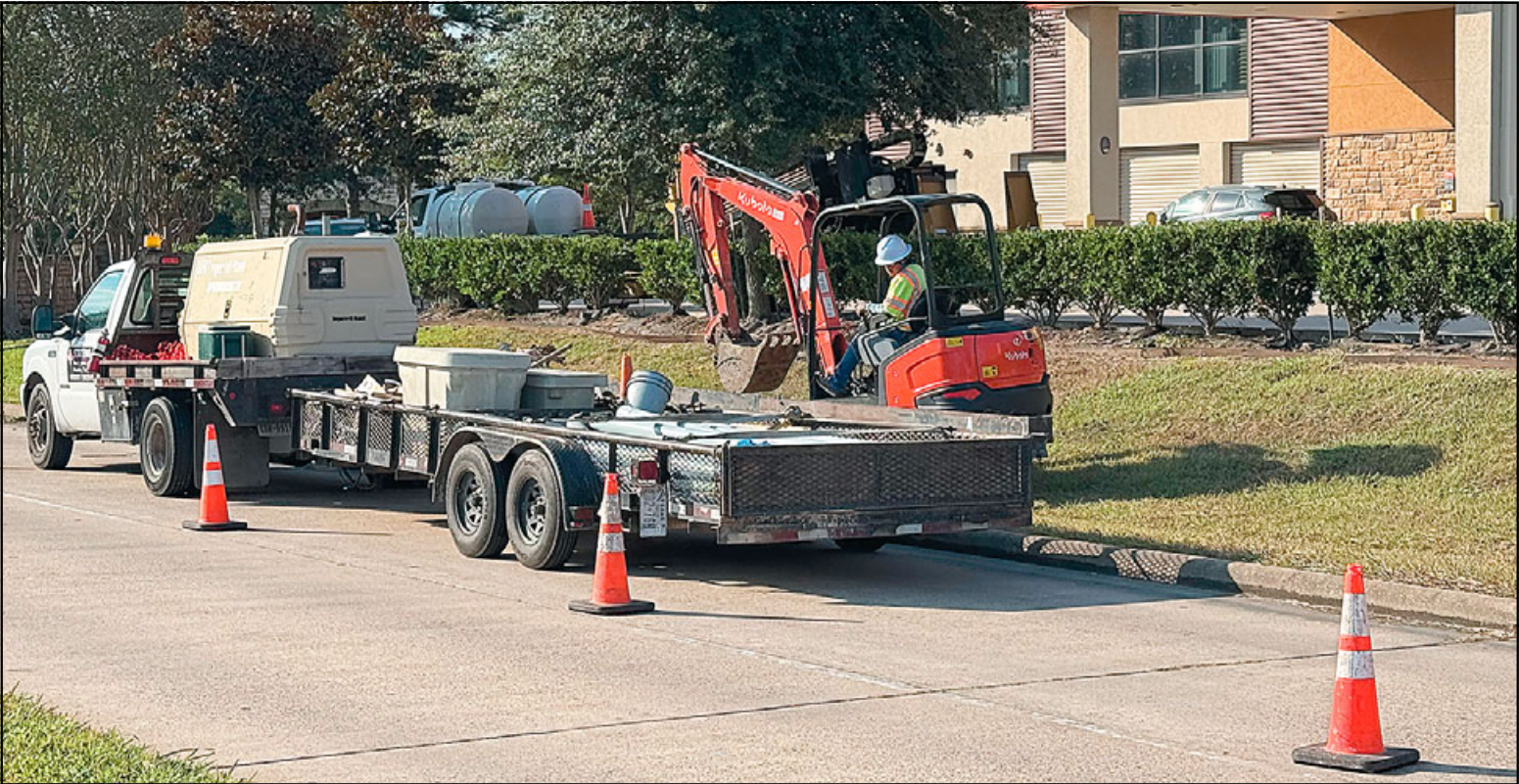
Construction related to a new traffic signal on Blackhawk at Riverstone Ranch Drive caused a gas leak the afternoon of Friday, Aug. 28. A subject of debate for nearly a decade, the signal is aimed to reduce traffic congestion at the intersection, which has become noticeably worse since the recent expansion of nearby Gateway Academy charter school.
