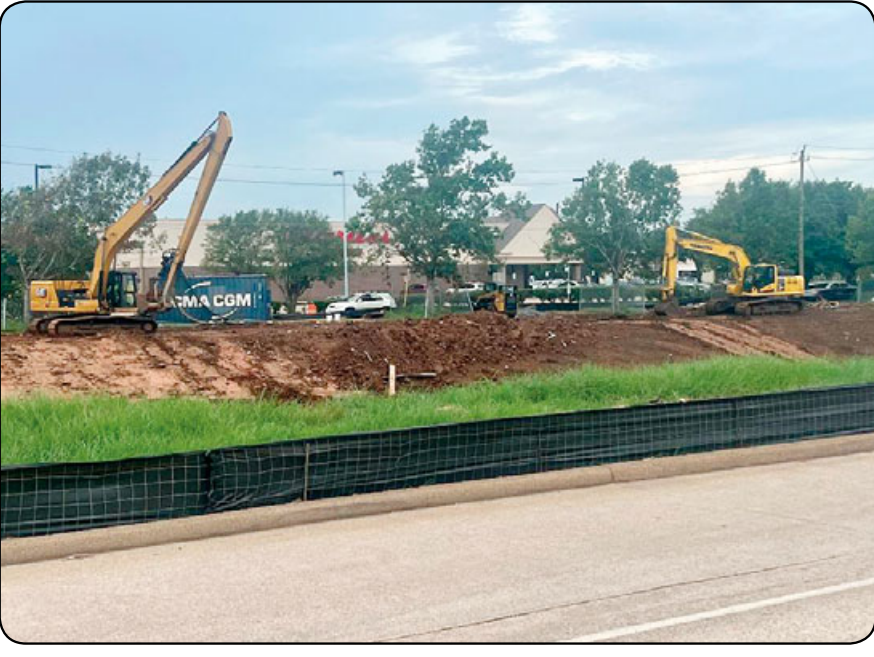
Work continues on the Harris County project to make drainage improvements to the Beamer Ditch. Construction was to be broken into three phases. Phase 1 runs from Sagerock to Scarsdale; Phase 2 runs from Scarsdale to Astoria; and Phase 3 runs from Astoria to near Dixie Farm Road. Now in its final phase, work is expected to be complete by the end of the year. Photo by James Bolen
