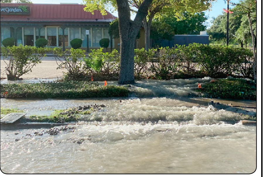
Broken water pipes forced the closure of the Olive Garden restaurant in the 12700 block of the Gulf Freeway near Fuqua both Friday, Aug. 11, and Saturday, Aug. 12. Local officials said water service the surrounding communities was unaffected, as the damage was believed to have been isolated to just that one business.
