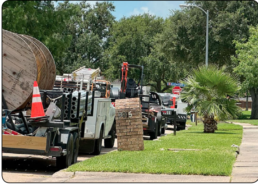
CenterPoint had contractor crews working on various electrical outage problems throughout last week. Approximately 80 households were affected near Blackhawk and the Sagemark area. Outages lasted off and on all last week from Sunday, until Saturday, June 29. Photo by Marie Flickinger
