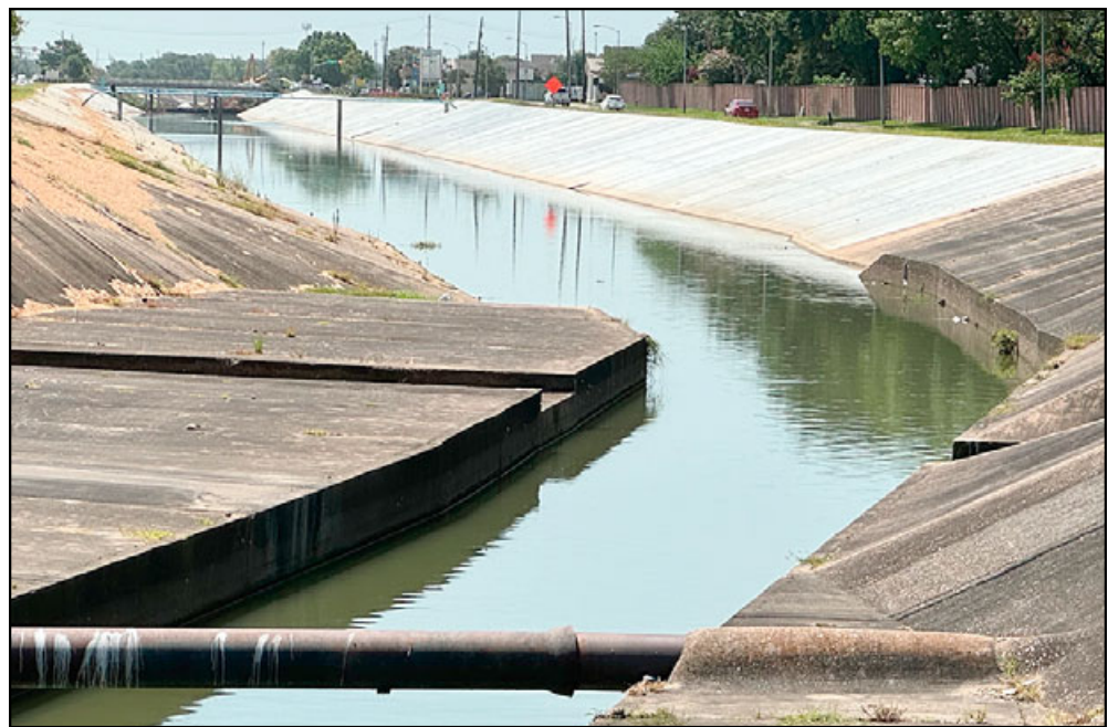
As work continues on the Beamer Road ditch, residents have called the Leader concerned about the constant standing water in the ditch. This is a result of construction in the ditch which necessitates blocking part of the ditch during construction. If a heavy rainfall were to occur, the blockage would be opened so the drainage could flow properly. The estimated time for completion of the ditch is scheduled for early this fall. Photo by Marie Flickinger
