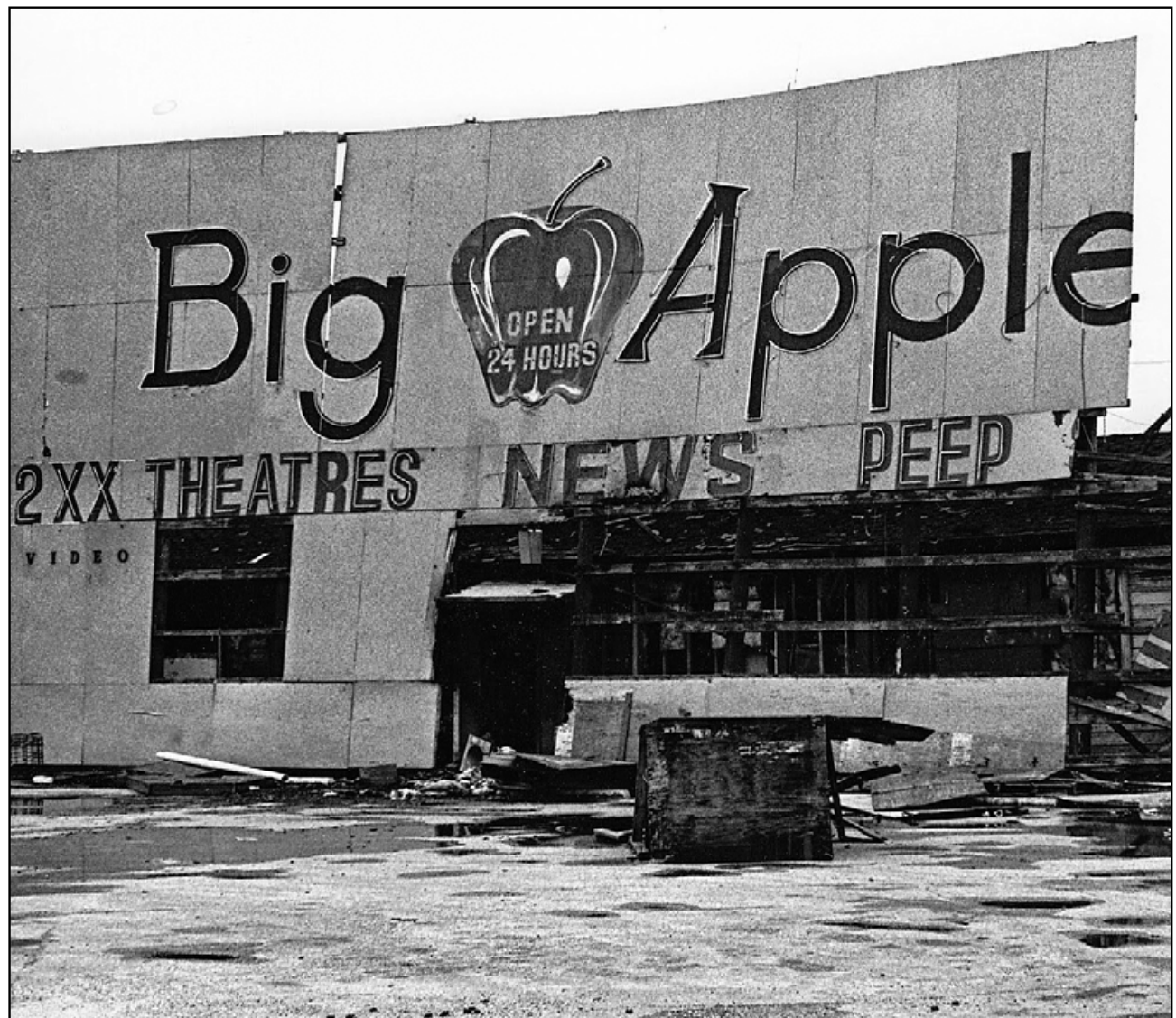
The building that once housed the controversial Big Apple adult theater on the Gulf Freeway near Edgebrook was recently leveled by demolition crews. Although the business has been closed for approximately 40 years, it was once deemed a scourge of the South Belt and opposed by several community leaders, who saw the pornographic establishment as unfit for the burgeoning family area. The former building is shown above after being damaged by a tornado associated with Hurricane Alicia in 1983. The business was destroyed by a suspicious fire two years later. Photo courtesy of South Belt Houston Digital History Archive. See related photos on Page 1 and Page 2.
