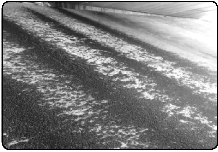
A colony of hundreds of bats has recently been spotted living under the bridge at Scarsdale and Beamer. The winged creatures leave behind large amounts of excrement under the bridge (shown above). Known in Spanish as guano, the excrement is often used as fertilizer because of its high content of nitrogen, phosphate and potassium – nutrients essential for plant growth. See related story and photos on Page 1A. Photo by Ronnie Thomas
