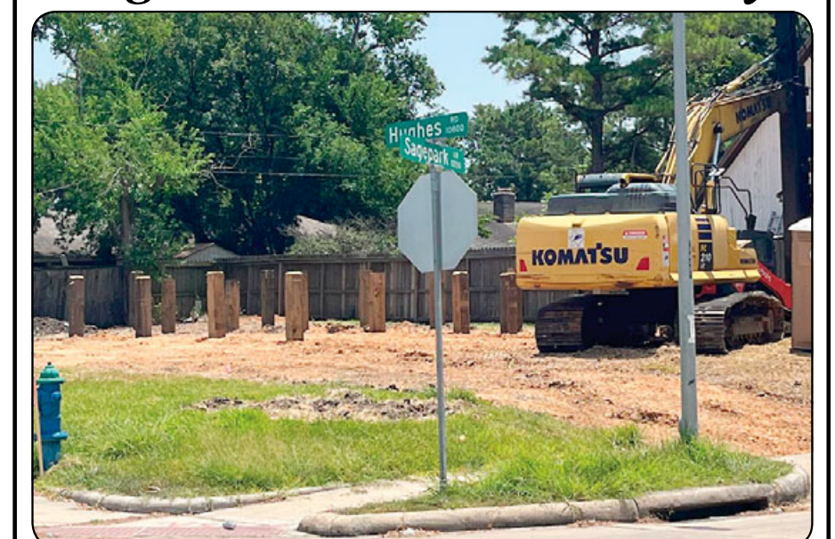
Construction recently began on Sagemont at Hughes Road to replace a home destroyed by Hurricane Harvey in 2017. The new replacement houses being constructed in the Sagemont subdivision show vast improvement over those initially proposed by the Texas General Land Office, which were smaller in size, had little to no brick and did not include garages.
