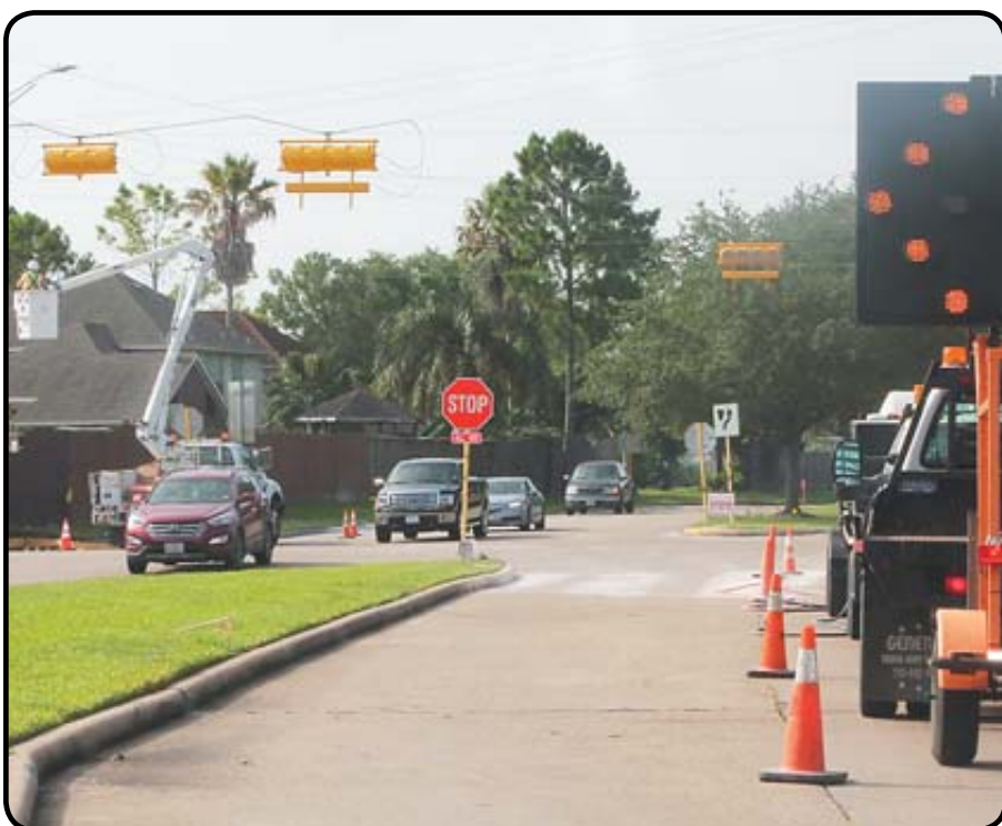
Harris County work crews are shown above installing a new traffic light at the intersection of Hughes Road and Blackhawk. County officials said the signal is needed to accommodate for future growth in the South Belt community. The $219,000 project is scheduled to be complete by the end of the month.
