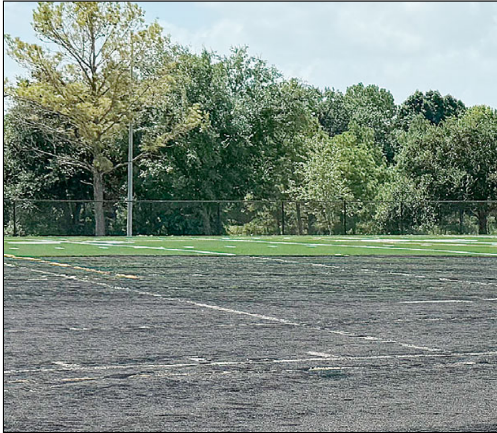
The turf covered athletic field for the Houston Gateway Academy located in Riverstone subdivision caught fire about 4 a.m. July 4. The school, which has been in some stages of planning since 2010, is finally nearing completion. The turf was installed last month. The fire destroyed about one-third of the turf. It was reported started by fireworks. Photo by Marie Flickinger
