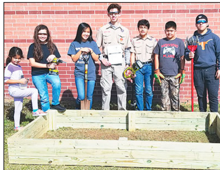
Eloy Sanchez Jr. (center) recently completed his Eagle Project as part of becoming an Eagle Scout. For his project, Sanchez constructed and installed two planter boxes at South Belt Elementary, his former campus. Helping Sanchez with the project were, left to right, Arianna Izaguirre, Aliyah Sanchez (Sanchez's sister), Victoria Chu, Daniel Garza, Arturo Izaguirre Jr. and Jacob Efird. Garza and Efird are also Scouts.
