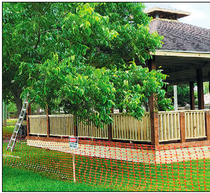
Clear Brook City MUD gazebos located at Bishop Park and Clear Brook City Park are undergoing repairs and upgrades. Both gazebos will not be available for use for the next 2-3 weeks as crews work to restore the structures.
