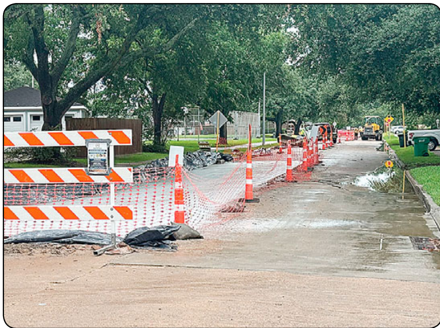
A Harris County construction project is currently underway near Sagemeadow Park to make street improvements. Traffic on Sageyork is currently in one direction only, with traffic from the other direction being detoured to Sagebud. Similar projects – being spearheaded by Precinct 2 Commissioner Adrian Garcia – are planned for the Highland Meadow, Wood Meadow and Sageglen subdivisions. Motorists are urged to use caution.
