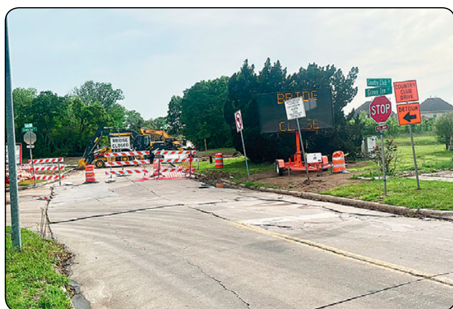
The bridge on Country Club Drive at Clear Creek near FM 518/Broadway in Pearland recently closed for a TxDOT replacement project that is expected to take approximately one year to complete. Other partners include the U.S. Department of Transportation and the City of Pearland. A temporary traffic signal was erected at Scarsdale and Bogey Way to alleviate additional congestion associated with the construction. Photo by James Bolen
