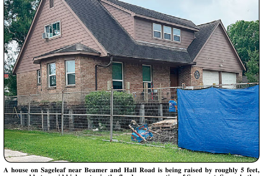
A house on Sageleaf near Beamer and Hall Road is being raised by roughly 5 feet, presumably to avoid high water in the flood-prone portion of Sagamont. Several other properties in the area have been purchased as part of county buyouts due to repeated flooding. At least one home in the area was rebuilt by the state following Hurricane Harvey. Photo by David Flickinger
