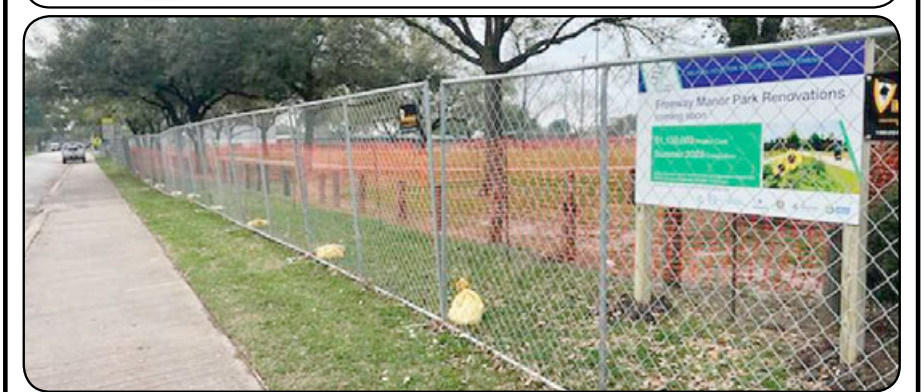
Freeway Manor Park is currently closed while city crews work on a construction project to make improvements to the aging park's baseball field, picnic areas, tennis courts, parking lot, walking trail, soccer field, benches, lighting and playground (shown in artistic rendering). The project is part of the city's 50/50 Park Partners initiative, which will make improvements at 11 area parks. The park is expected to reopen in June.
