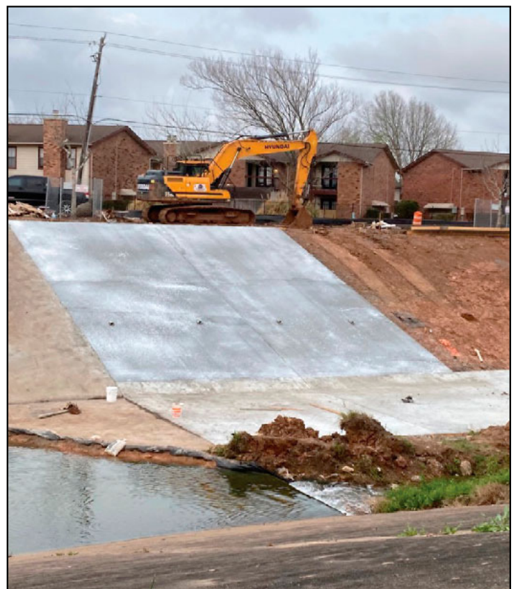
The Harris County Flood Control District recently began work on a massive project to make drainage improvements along the Beamer Ditch. The endeavor will provide concrete lining on the area ditch from Sagerock to near Dixie Farm Road. The project will be broken down into three phases. Phase 1 will run from Sagerock to Scarsdale; Phase 2 will run from Scarsdale to Astoria; and Phase 3 will run from Astoria to Beamer near the South Belt Stormwater Detention Basin. Construction of the $10.7 million project is expected to take approximately two years to complete. Photo by Marie Flickinger
