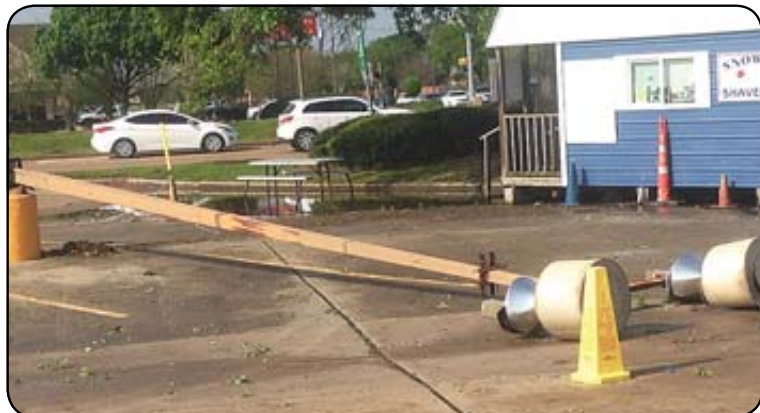
A steel light pole was snapped in half in the Food Town parking lot at Scarsdale and Beamer. Photo by James Bolen
