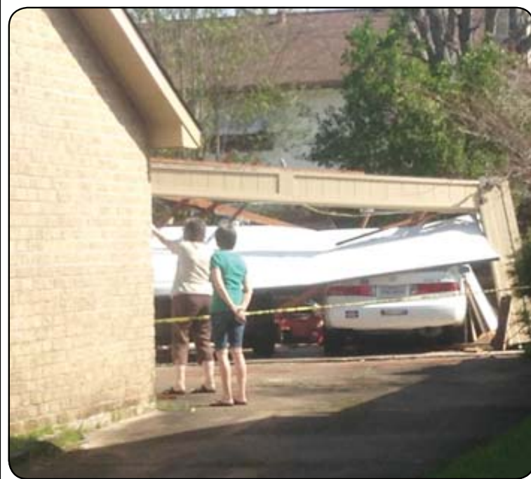
A neighbor comes to assess the damage of a collapsed garage at the home of George and Kathy Ericksen at 11607 Sagevale at Sagegreen. The damage was featured in a Channel 2 news report. Photo by James Bolen
