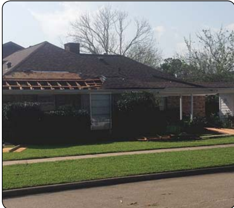
A roof was torn from a house at the corner of Sagegreen and Sagevale in the Sageglen subdivision, the intersection where the most significant damage was reported. Photo James Bolen
