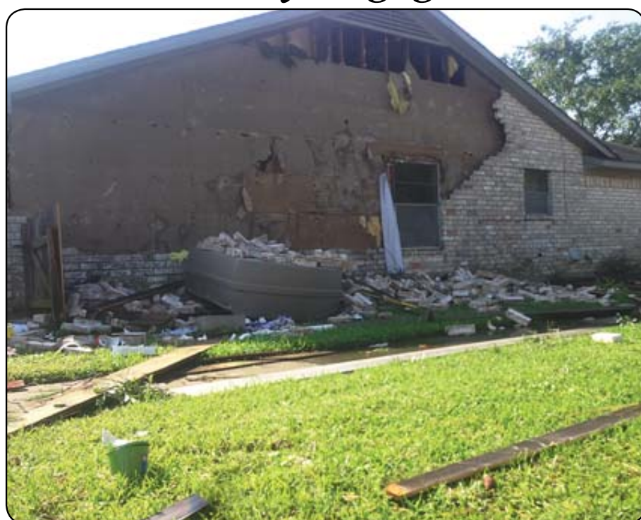
The South Belt community was hit hard by strong storms this past weekend, causing extreme damage to several area homes and businesses. The above residence is at the intersection of Sagegreen and Sagevale in the Sageglen subdivision, where the worst of the damage took place. Despite online reports to the contrary, the damage was not the result of a tornado, according to experts. See additional photos on Page 6A. Photo by James Bolen
