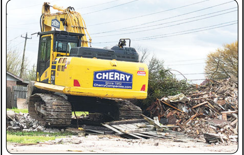
Houses in the Kirkmont and Scarsdale subdivisions, including the one shown above in the 9500 block of Sagebend, were recently demolished due to repeated flooding. According to Harris County Flood Control District officials, however, funding to level the homes was already secured before Hurricane Harvey and not related to the recent storm. The Leader is asking the resident who emailed a similar picture from Scarsdale to contact the paper, as the original message has been lost. Photo by Marie Flickinger
