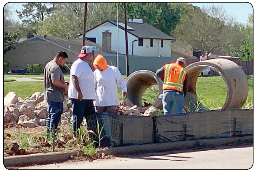
Work recently resumed on the county's Beamer Ditch project after being dormant for months when the original contractor abandoned the job. In January, Harris County Flood Control District selected Rebel Contractors as the construction company to complete the project. Complete Concrete was originally awarded the low-bid contract to widen the ditch and install concrete lining from Sagerock to near Dixie Farm Road. Photo by Marie Flickinger
