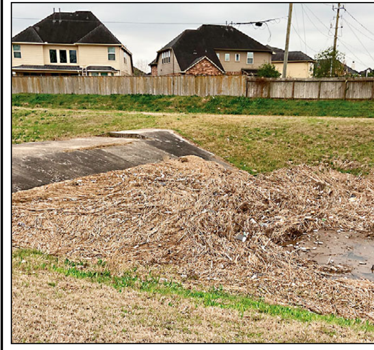
The above photo was taken by Amanda Maslonka along the South Belt Hike & Bike Trail. The Leader contacted Harris County Flood Control officials who agreed to clean up the debris to promote proper drainage. Additional photos taken by the Leader show considerable trash in the drainage area, including a window unit air conditioner. The Leader thanks Maslonka for interest in improving drainage in the community.
