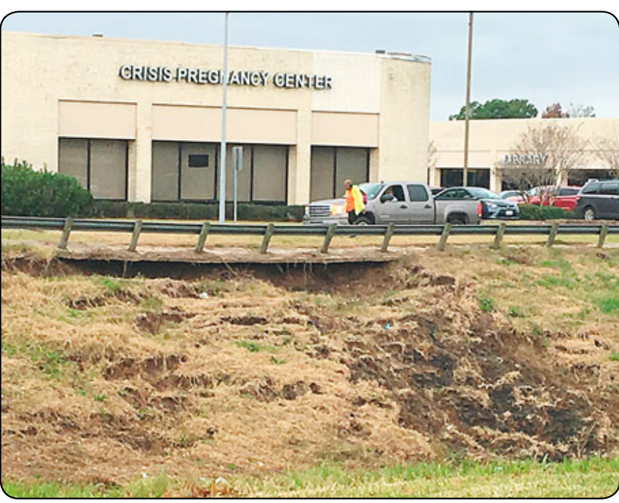
Ground erosion along the Beamer ditch has caused a guardrail to collapse, worrying many drivers who question the stability of the adjacent street. County officials have inspected the problem and determined it is not an immediate threat, as the erosion has yet to go beneath the roadway. Nevertheless, it has been marked as an emergency repair and will be addressed in the near future. See related photo on Page 6A. Photo by David Flickinger
