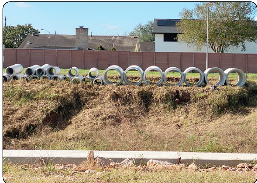
The Mud Gully Channel Conveyance Improvements Project, also known as the Beamer Ditch Project, is scheduled to go before Commissioners Court Dec. 13, the lone court meeting this month due to the Christmas holidays. Abandoned by the original contractor this past February, the project must now be reauthorized by Commissioners Court before moving forward. Concrete piping is shown above at the dormant site. Photo by Marie Flickinger
