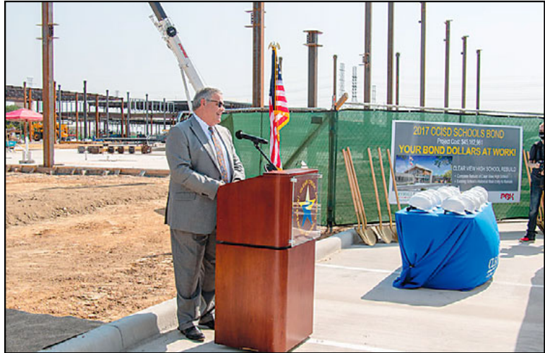
Superintendent Dr. Greg Smith gives his remarks at the Oct. 13 groundbreaking of the rebuild of Clear View High School with the rudimentary structure of the new high school seen in the background.
