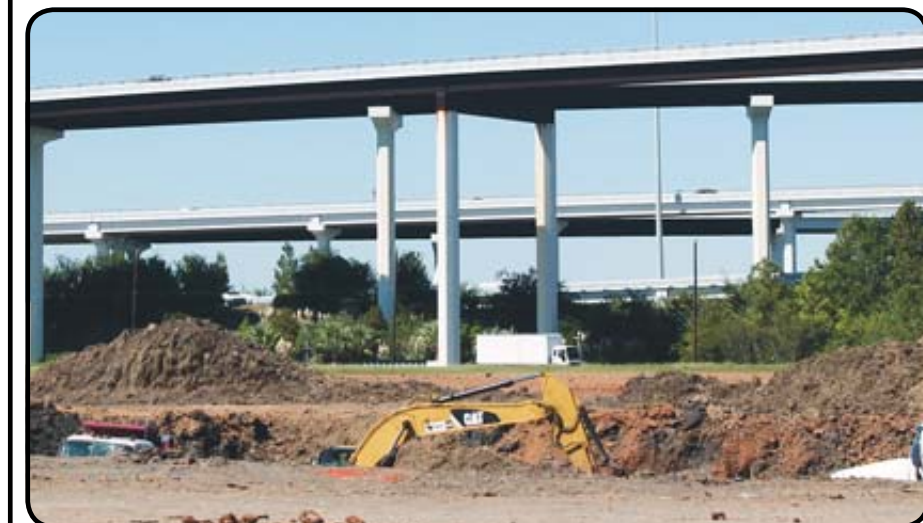
Construction recently began on a new recreational vehicle park at the southwest corner of the Gulf Freeway and Beltway 8, just east of the Sagemont subdivision. Workers are shown above digging a pond on the 13-acre site. To put the pond's depth in perspective, one of two large trucks is barely visible. The Big Spot RV Resort is scheduled to open by April 1. Photo by Marie Flickinger
