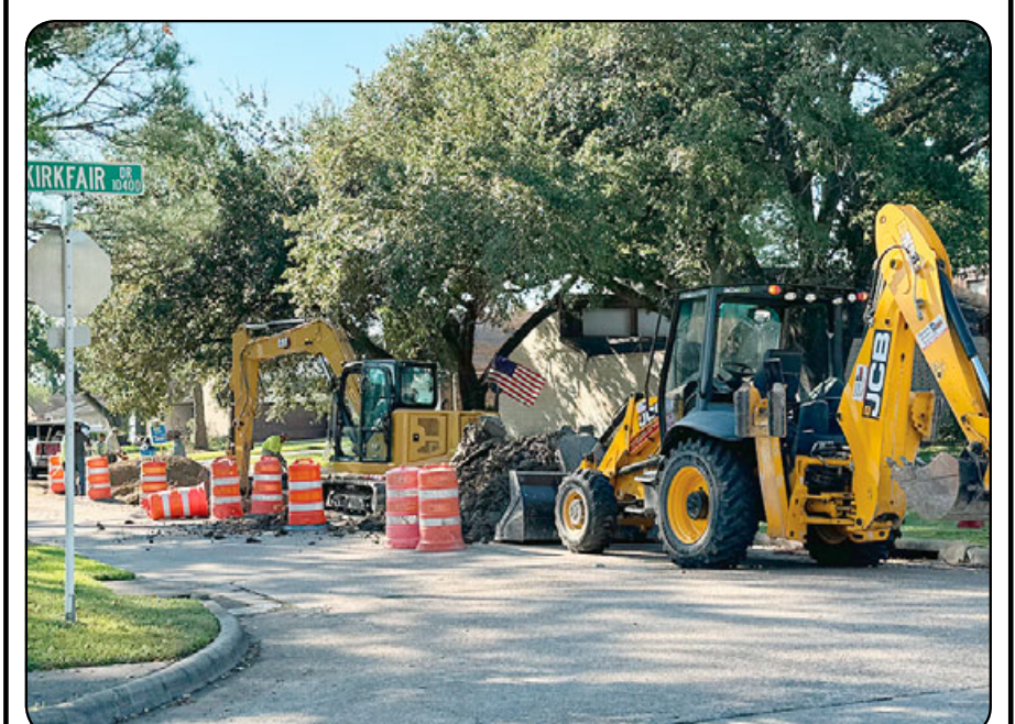
Local commuters in the Kirkwood South subdivision have undoubtedly encountered multiple ongoing construction projects in the community. Harris County crews are undertaking multiple road improvement projects in the area subdivision simultaneously, as shown above on the Kirkfair thoroughfare. Photo by David Flickinger
