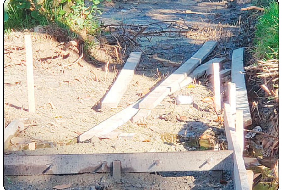
Multiple residents have contacted the Leader in recent weeks, concerned about sidewalks near Sageriver being in disrepair following city work done on nearby streets. While the street construction was completed, work on the sidewalks was not, causing safety hazards and eyesores. After repeated calls to the contractor, Michael Kennedy of TLC Engineering told the Leader that work on the sidewalks would begin Tuesday, Oct. 16, weather permitting, and take roughly 10 days to complete. Kennedy said rainy weather caused the delays. Photo submitted by Lynn Medeiros
