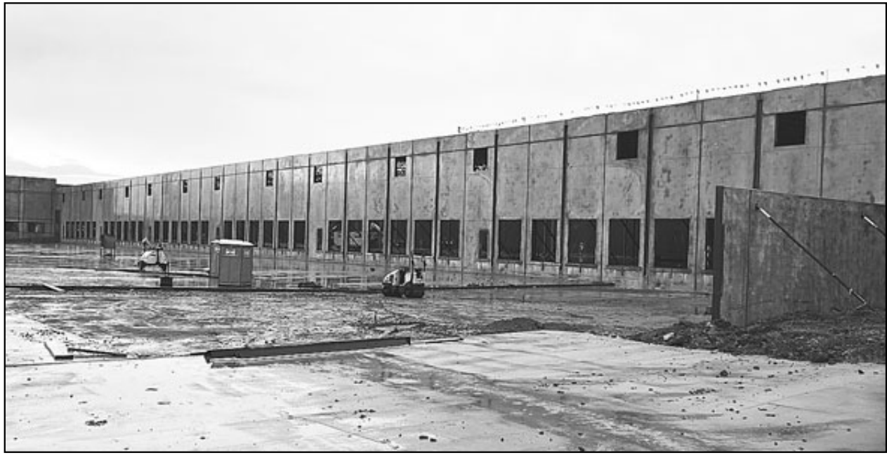
Vigavi Realty developers is constructing a 170,000-square-foot facility for a front load distribution center at 730 Genoa Red Bluff Road. The project is being constructed on 10+ acres and includes 37 dock doors. The facility is nearing completion. It includes 51 trailer stalls and two drive-in ramps with a clearing height of 32 feet. It is designed to serve as a heavy distribution center. Photo by Marie Flickinger
