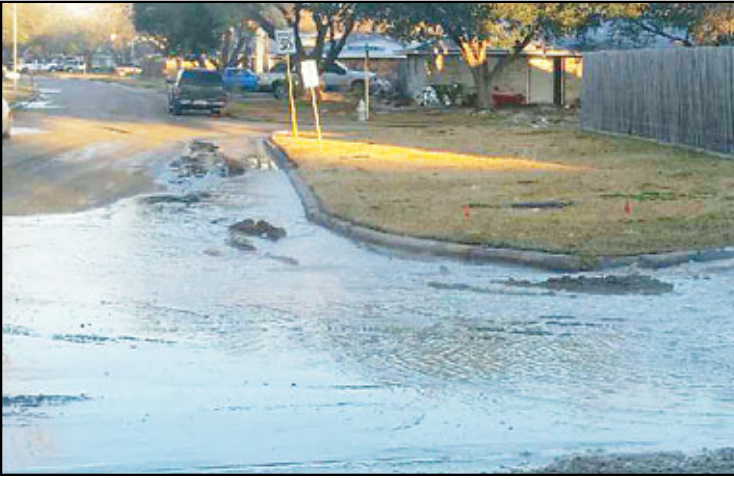
A pipe ruptured at a City of Houston force main located on Scarsdale at Brookmeadow on Tuesday, Jan. 16. Crews were unable to immediately shut down the facility, as it provides service for the nearby hospital.
