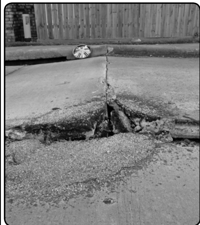
Several South Belt residents have complained in recent weeks about a buckle in the road on Sabo between Sagetree and Sageforest, presumably caused by the ongoing drought. The above photo, taken by Kirkwood Civic Club President Ralph Robbins, shows a hubcap that fell off due to the damage. The street has since been repaired by the city.
