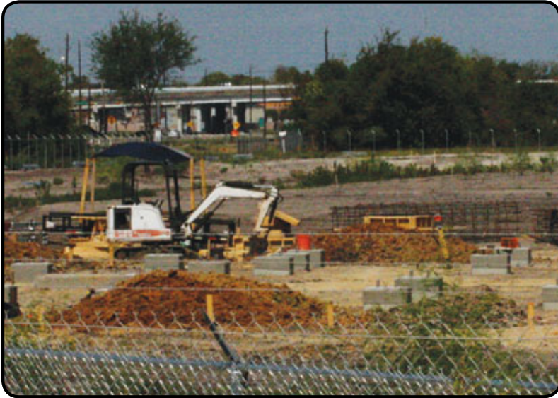
Enterprise Products Partners is currently constructing a crude oil storage facility on 150 acres of land along Highway 3 between Beltway 8 and FM-2553 (Scarsdale). Due to open for business in mid-2012, the terminal will connect local refineries to ongoing production in South Texas via the Seaway Pipeline. See related story on Page 2A.
