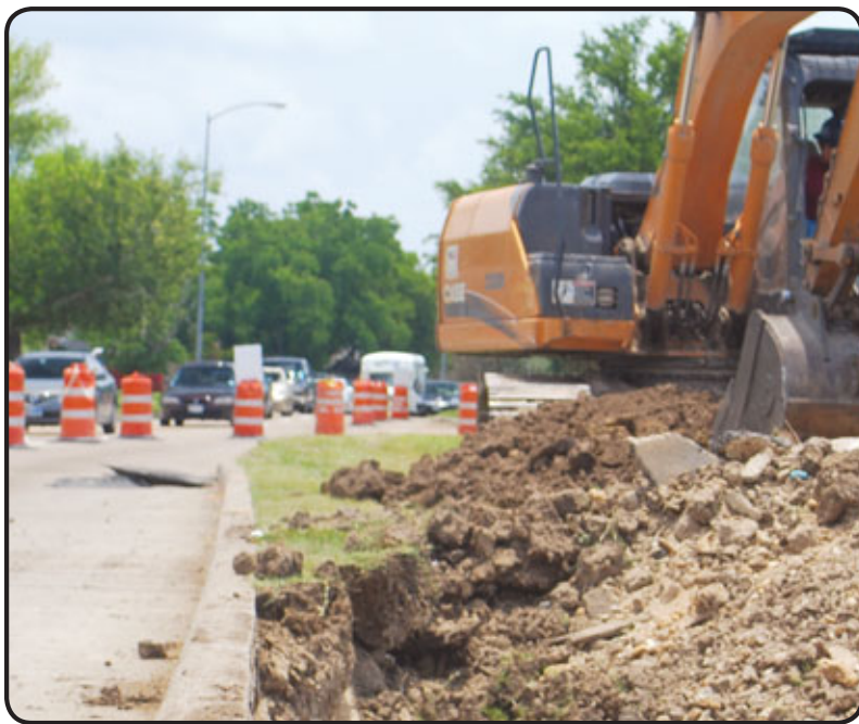
Construction began Tuesday, June 1, on Blackhawk south of Beltway 8 to build a left-turn lane that will head toward Highway 288. Construction is expected to take roughly 80 days to complete. Affected residents are urged to take alternate routes if possible to avoid congestion at the intersection. A right-turn lane that heads toward the Gulf Freeway will be constructed at a later date. The Leader has been working with Harris County Precinct 1 Commissioner El Franco Lee for roughly four years to get the work done. The South Belt-Ellington Chamber of Commerce and the Harris County Precinct 2 Constable's office also played an integral role in the process.
