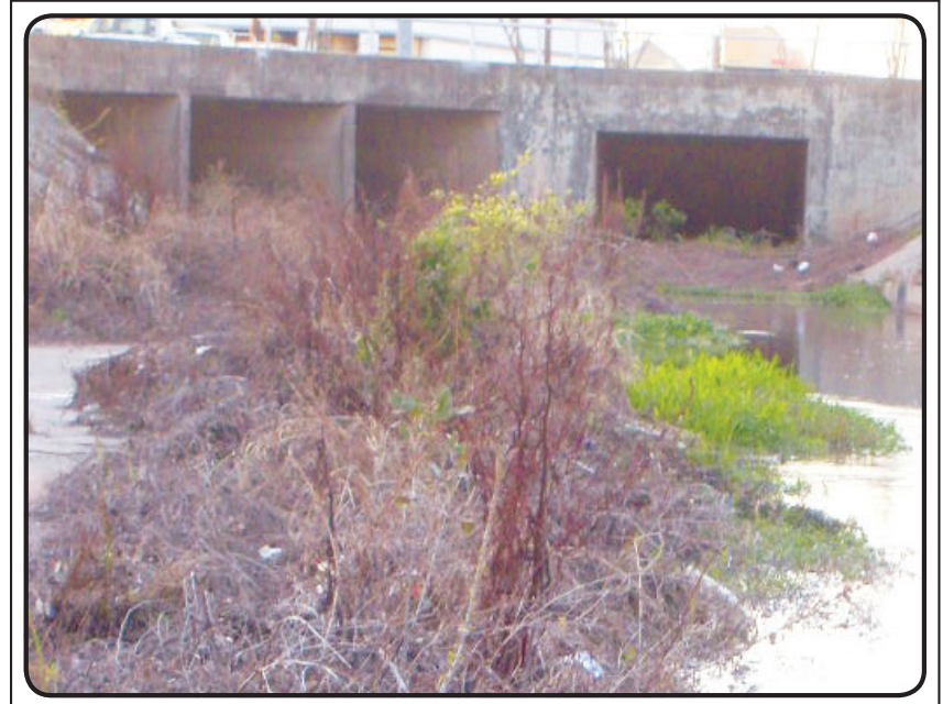
Sagemont resident Florence Frey is on a mission to have the ditch on Beamer near Hall Road cleaned of silt and vegetation. Frey's house has flooded twice, and she feels the inefficient drainage system was largely responsible. The last time the Harris County Flood Control District desilted the bayou was in 2002. Photo by Frey's daughter, Monica Eaton
