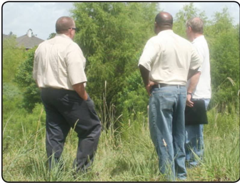
The vegetation in the ditch that runs through Clear Brook Meadows has grown above the banks and is causing drainage issues. From left, David Matthews from Harris County Precinct 1, Curtis Lampley from the Harris County Flood Control District and Chris Clark of Clear Brook City MUD examine the trees and other plants growing in the ditch. The ditch has not been cleaned out because until recently, it was unclear as to whether the area is considered a wetland in the eyes of the U.S. Army Corps of Engineers.
