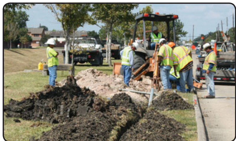
Construction crews are shown above installing fiber optic cable along Beamer near Scarsdale. The new cable will connect to the Houston Transtar system, allowing lights from Beltway 8 to Dixie Farm Road to sync up, which in turn will lower vehicle emissions. The Harris County Precinct 1 project, referred to as congestion mitigation and air quality (CMAQ), also received state and federal funding.
