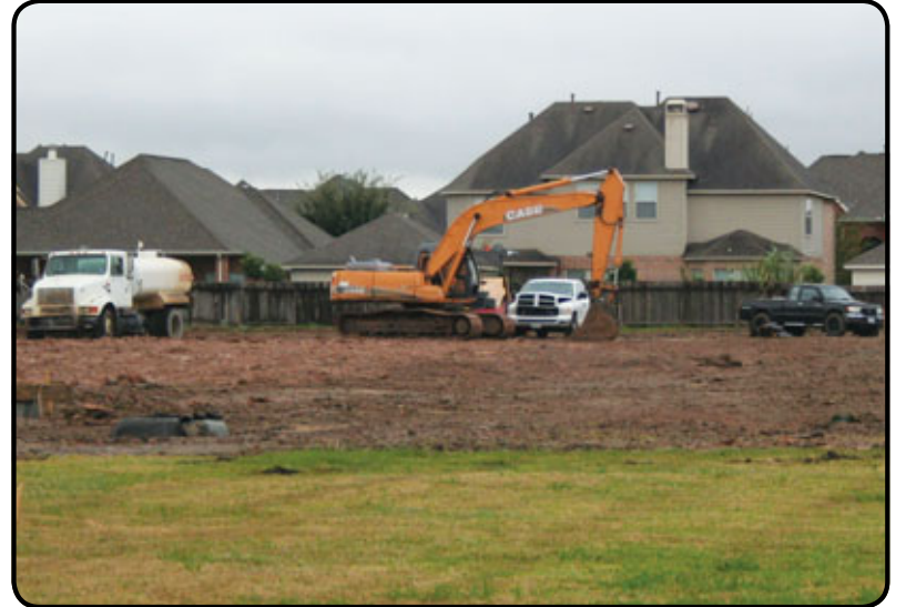
Construction recently began on a new skilled nursing facility to be located on Beamer at Scarsdale near Memorial Hermann Southeast Hospital. Clear Brook Crossing Rehabilitation & Healthcare Center will offer short-term rehabilitation as well as long-term care services, according to company spokeswoman Darcy Whatley. The facility is scheduled to open November 2012. Work crews are shown above clearing land for the center. Photo by David Flickinger
