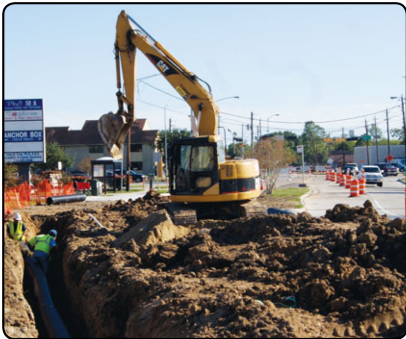
Construction continues on the stretch of Sabo Road between Kingspoint and Fuqua. Part of the City of Houston's Capital Improvement Plan (CIP), the project will replace existing storm drainage and pavement. According to the city's Public Works and Engineering Department, the estimated cost of construction is $4 million. Photo by James Bolen
