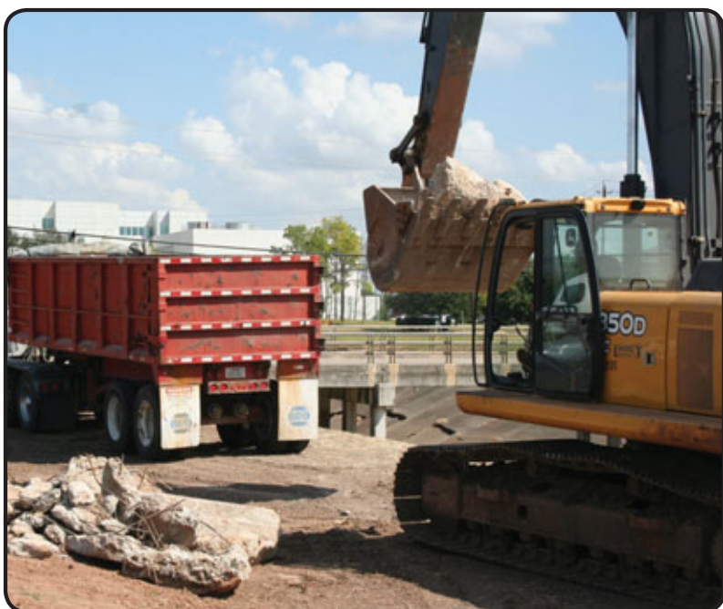
The Harris County Flood Control District recently began cleaning and repairing the Beamer ditch from Dixie Farm Road to Hall Road. Crews are shown above at Beamer and Astoria excavating concrete to be replaced. In all, 2,650 feet of the ditch are to be demolished and repaired. The work is scheduled to be complete in November, weather permitting.
