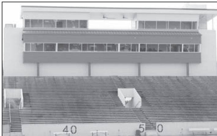
Contractors completed work of the revamped press box at Veteran's Memorial Stadium in Pasadena just in time for the start of the 2008-2009 athletic schedule. Improvements included an elevator and more space for working personnel. Additional seating was also placed for both press box and special visitor usage.
