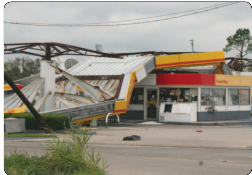
The South Belt area was hit hard by Hurricane Ike early morning Saturday, Sept. 13. Nearly four months later, residents are still recovering from the damage caused by the storm. Shown above is the Shell station at Scarsdale and Interstate 45, which suffered extreme damage when a power line fell on it, crushing its carports.
